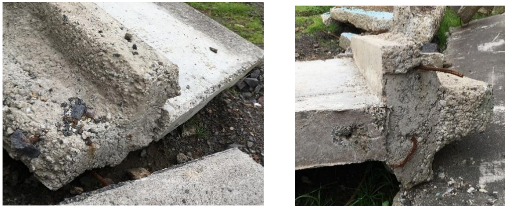
Figure 23: College Road floodwall - Views of the ends of two of the wall sections, showing the subsurface keys (Source: Bay of Plenty Regional Council, 2017)
